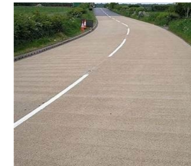
High Friction Surfacing on Road
