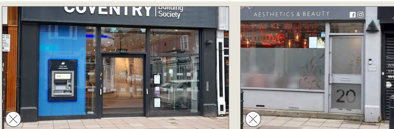
Left and right: These shopfronts appear to have lost their historic entrances and present a flat presence to the street with no depth to the entrance sequence. They have also likely lost original materials or details as a result.
