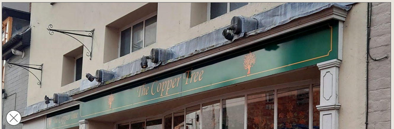
Top left, top right and above: Internally illuminated signage, exposed trough lights and exposed spotlight fittings will not be supported.
